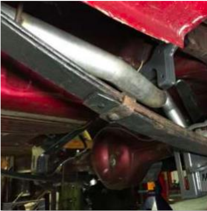
F – Reference photo of completed installation
