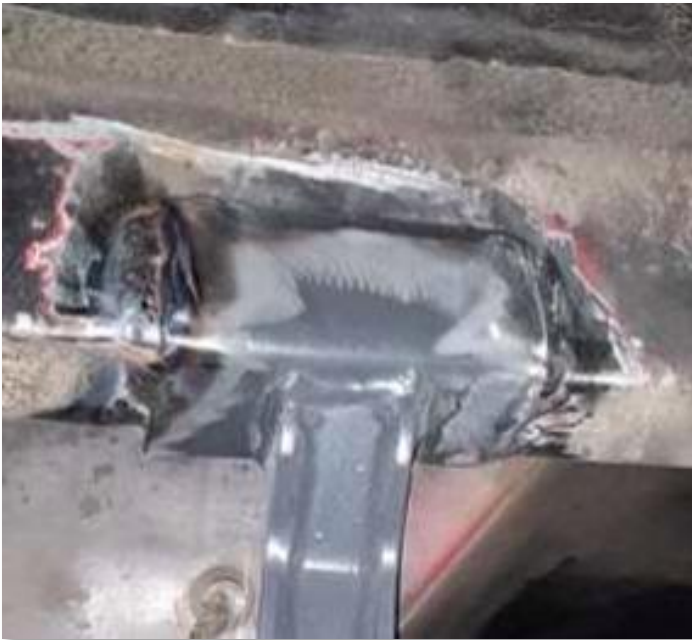
D.2 – Passenger's side of bracket, stitch welded to the frame rail
